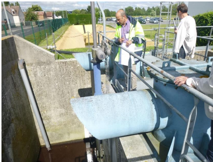
Figure 2-5 : Station de pompage de SANOFI
